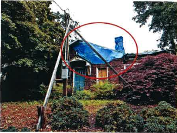
Location of fallen brick at front façade
