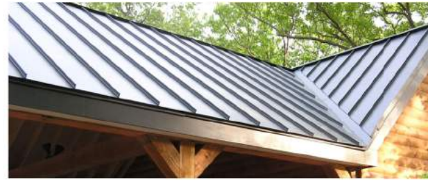
STANDING SEAM METAL ROOF - REAR PORCH ROOF SHEFFIELD METALS COLOR: CHARCOAL GRAY
