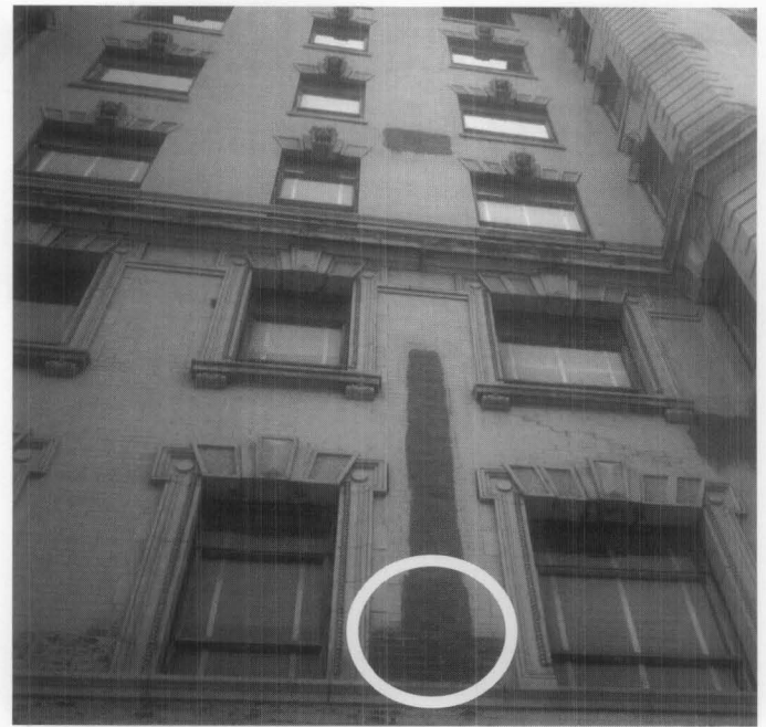
Figure 3. This small test area has revealed a red brick patch that does not match the original beige brick. This may explain why the building was painted, and may suggest to the owner that it may be preferable to keep it painted.
