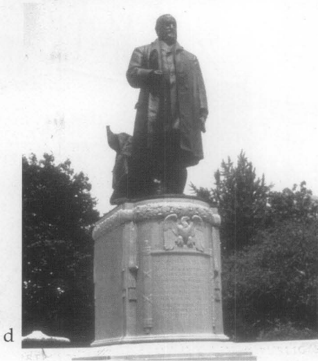
Figure 16. (a) The limestone base was heavily stained by runoff from the bronze statue above. (b) A poultice consisting of copper stain remover and ammonia mixed with fuller's earth was applied to the stone base and covered with plastic sheeting to keep it from drying out too quickly. (c) As the poultice dried, it pulled the stain out of the stone. (d) The poultice residue was removed carefully from the stone surface with wooden scrapers and the stone was rinsed with water. Photos: John Dugger.
