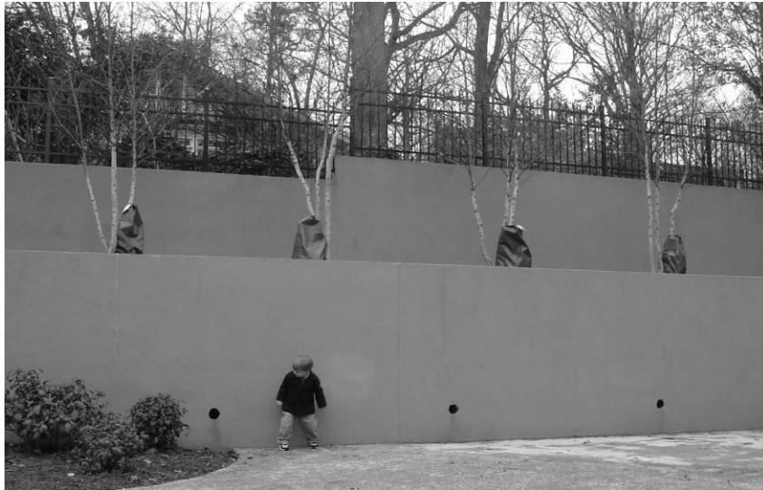
Large retaining wall on new construction that is out of scale with the built environment of Chelsea Heights.
