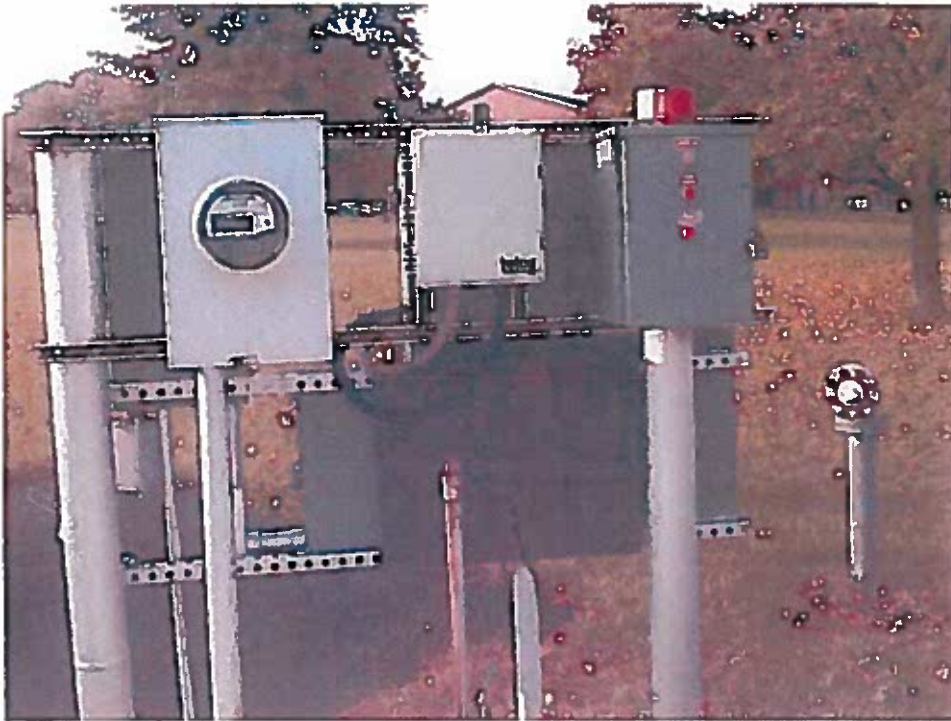
RS-33u monitoring a lift station
