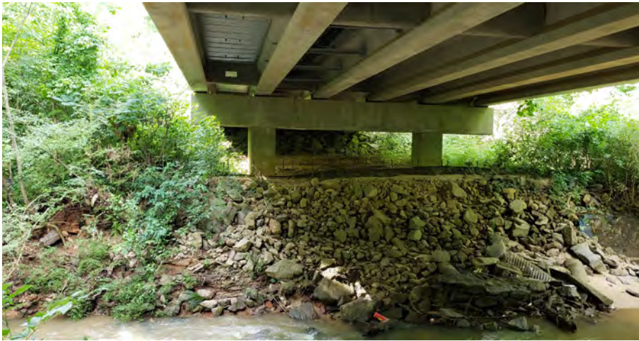
Existing conditions under Flowers Road, facing north. 8'-0" clearance for multi-use trail is achievable under Flowers Road
