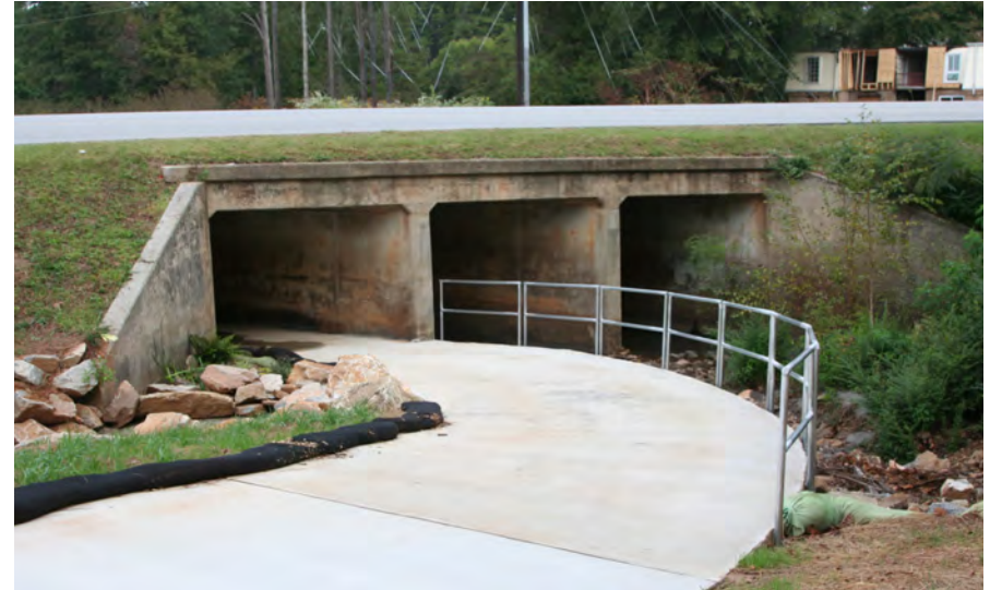
Multi-use trail going through an existing creek box culvert under a roadway.
