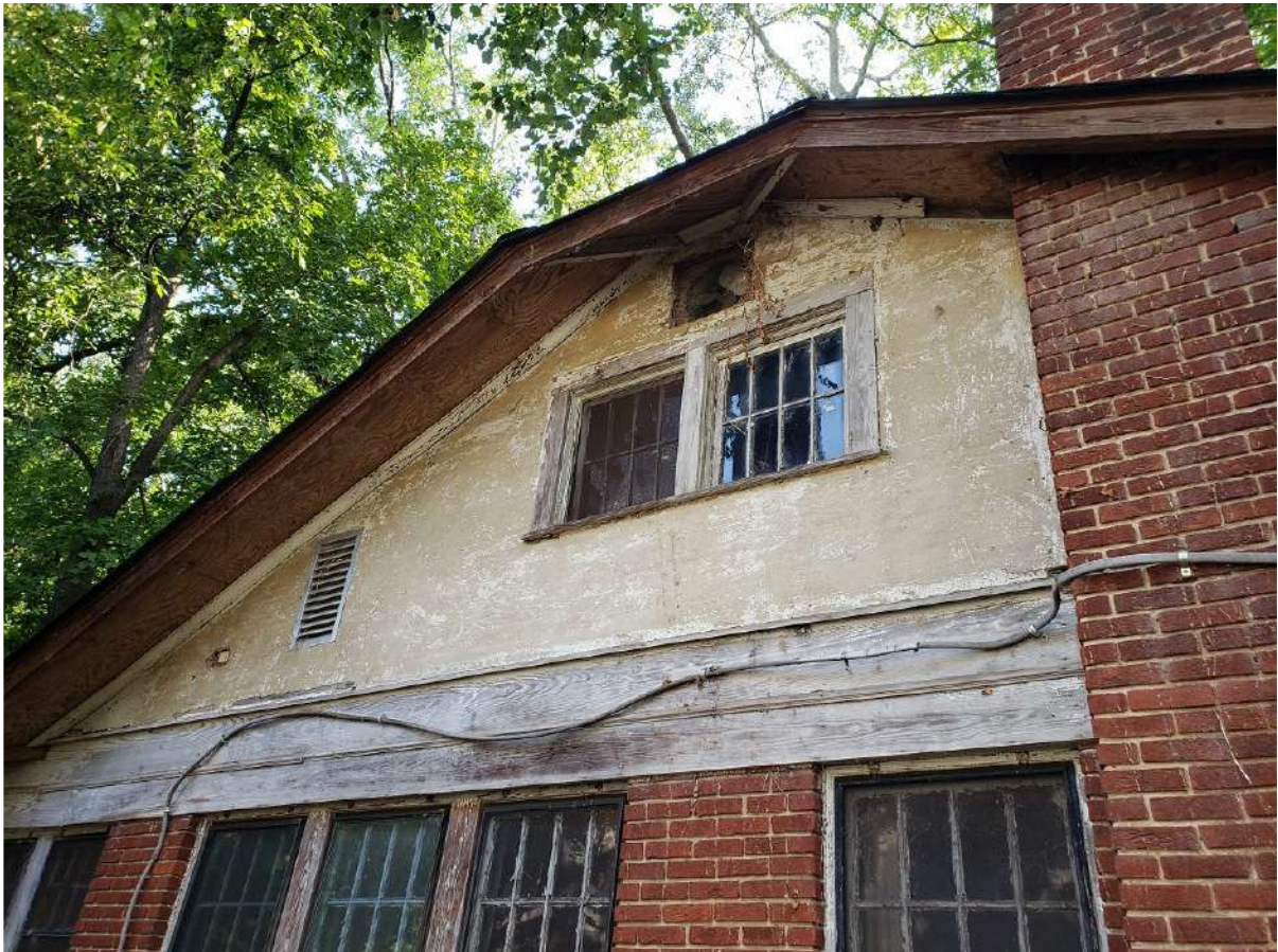
Left side showing fire damage and non-historic gable finish
