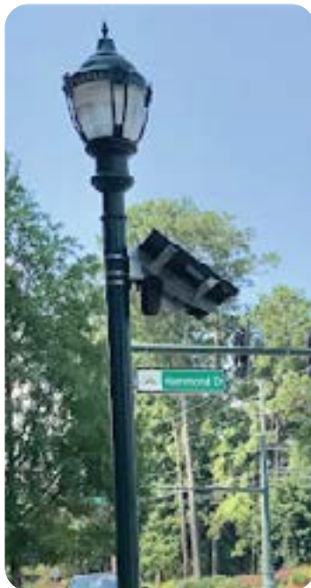
City intersection Solar & existing pole
