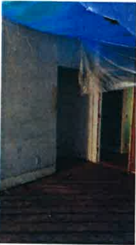
Demonstrating interior, exposed to the elements for two years after tree fell
