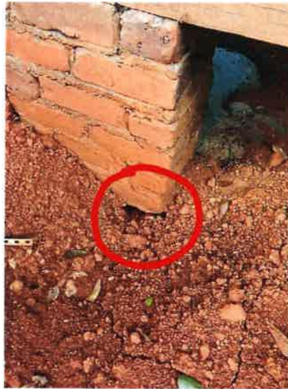
Figure 1 Void at bottom shows no footing
