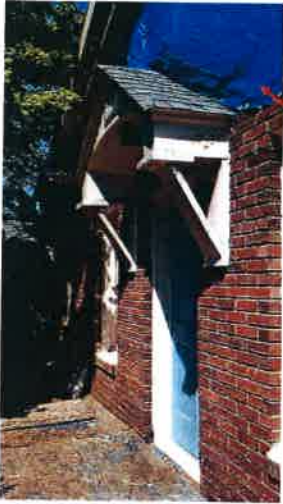
Location of fallen brick at front façade
