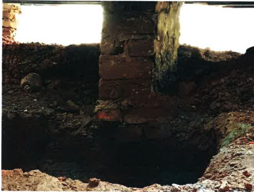
Figure 3 Excavation shows no footing for brick pilaster
