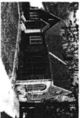
Some of the porch enclosures that detract from the overall integrity of the area.
