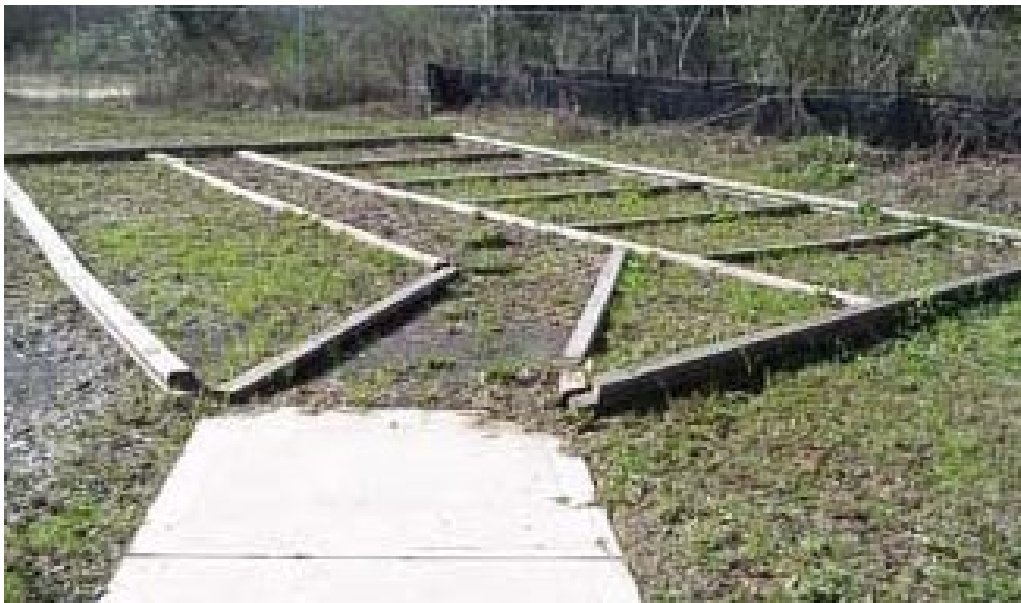
Not Acceptable No fence; overgrown with weeds.
