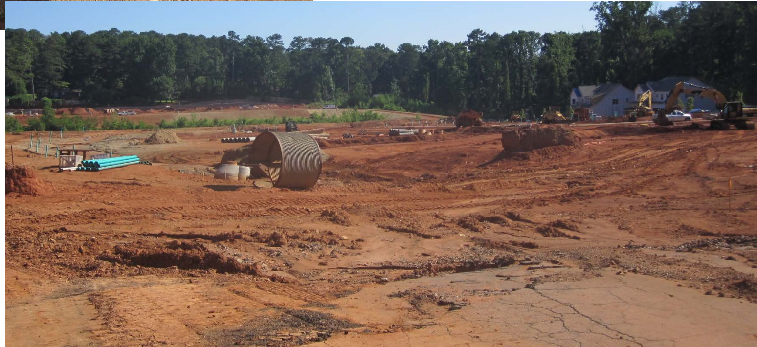
Rear of property where townhomes are proposed. Single-family homes can be seen at right side of photo.
