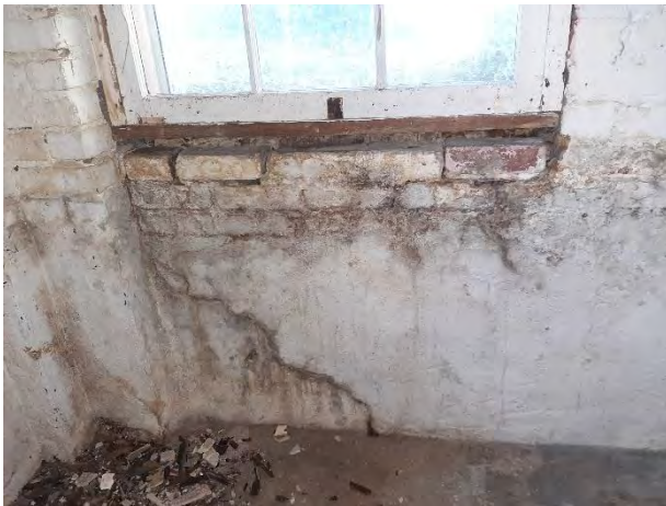
Photo 8 Stair-Step Crack at Basement
