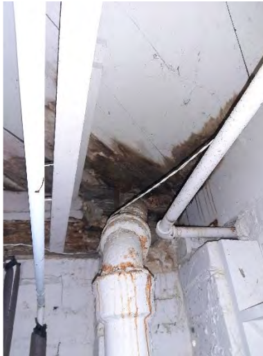
Photo 26 Floor Damage below Breakfast Nook
