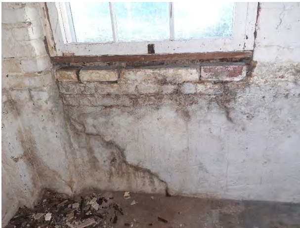
Photo 8 Stair-Step Crack at Basement
