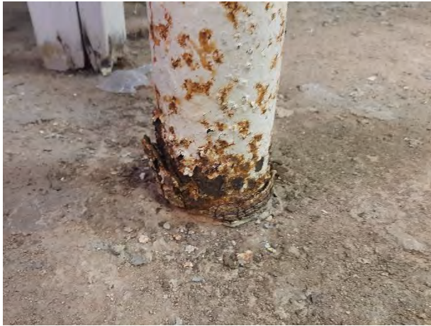
Photo 31 Rusted Bottom of Column
