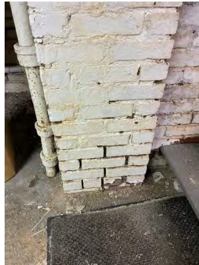
Photo 9 Loss of Mortar at Brick
