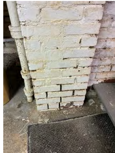
Photo 9 Loss of Mortar at Brick
