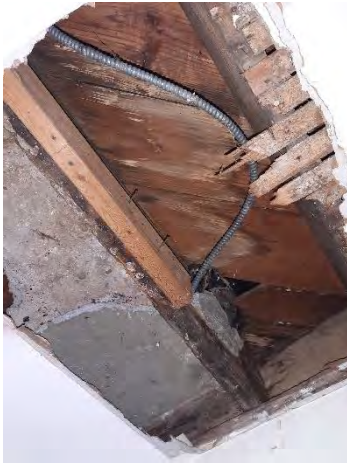
Photo 16 Damage at 2nd Floor Framing
