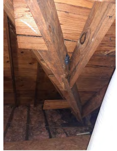
Photo 15 Dislodged Roof Rafter
