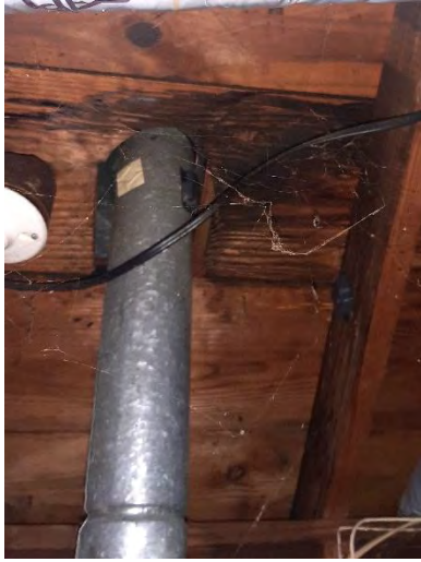
Photo 13 Water Damage at Vent
