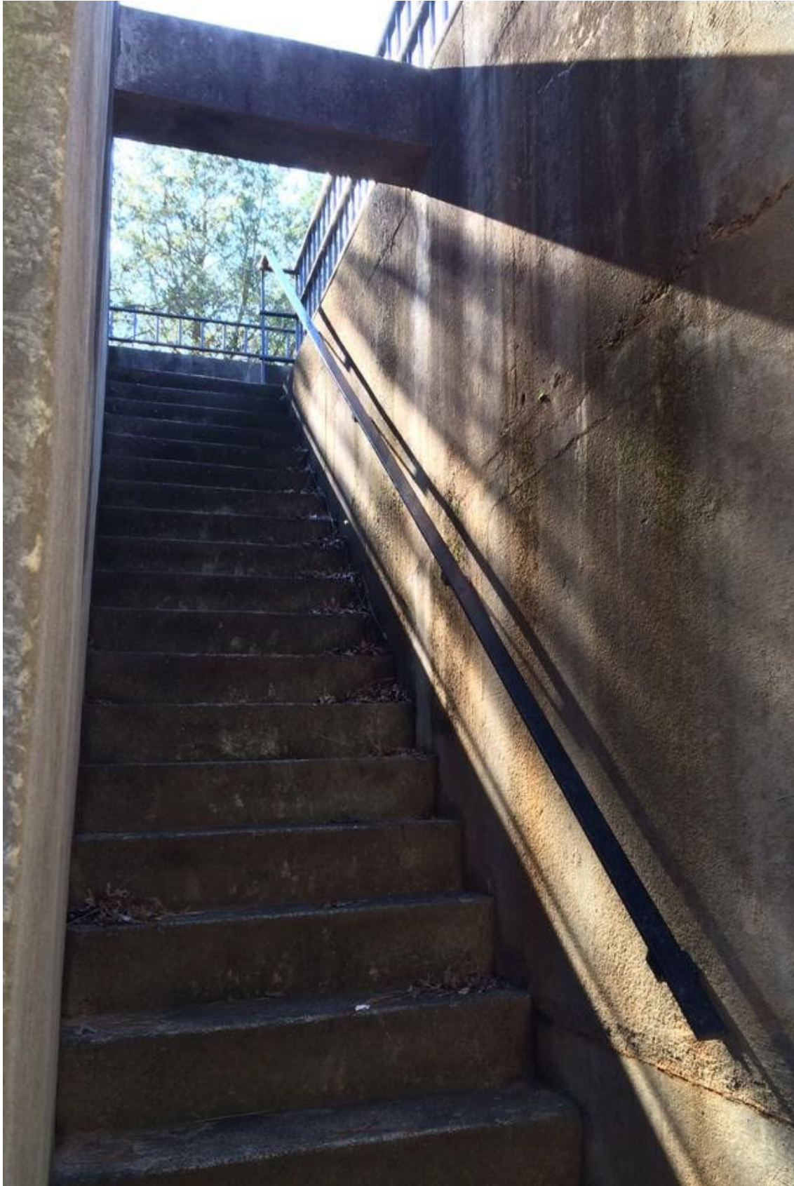
Here's the view from the stairwell. A pile of leaves and other trash sit at the foot of it.
