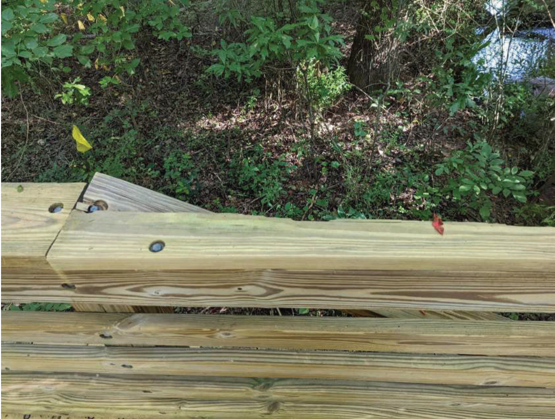
Photo 9 – Boardwalk Handrail Cap Broken (Split Lengthwise)
