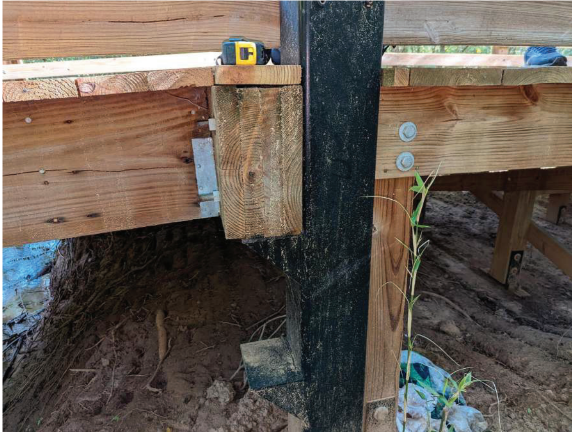
Photo 4 – Bridge #1 Quadruple End Beam & Steel Post Connection
